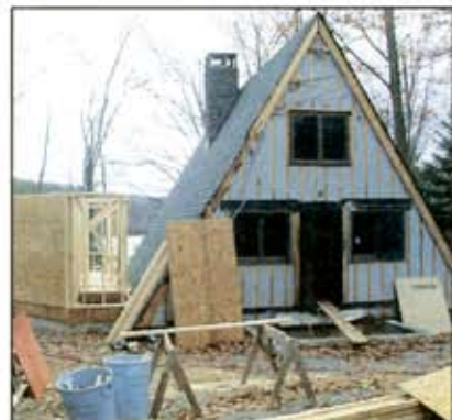
Clemleddy Construction adds living and storage space to what was once a seasonal home and upgrades the structure's heating and electric systems and insulation.
